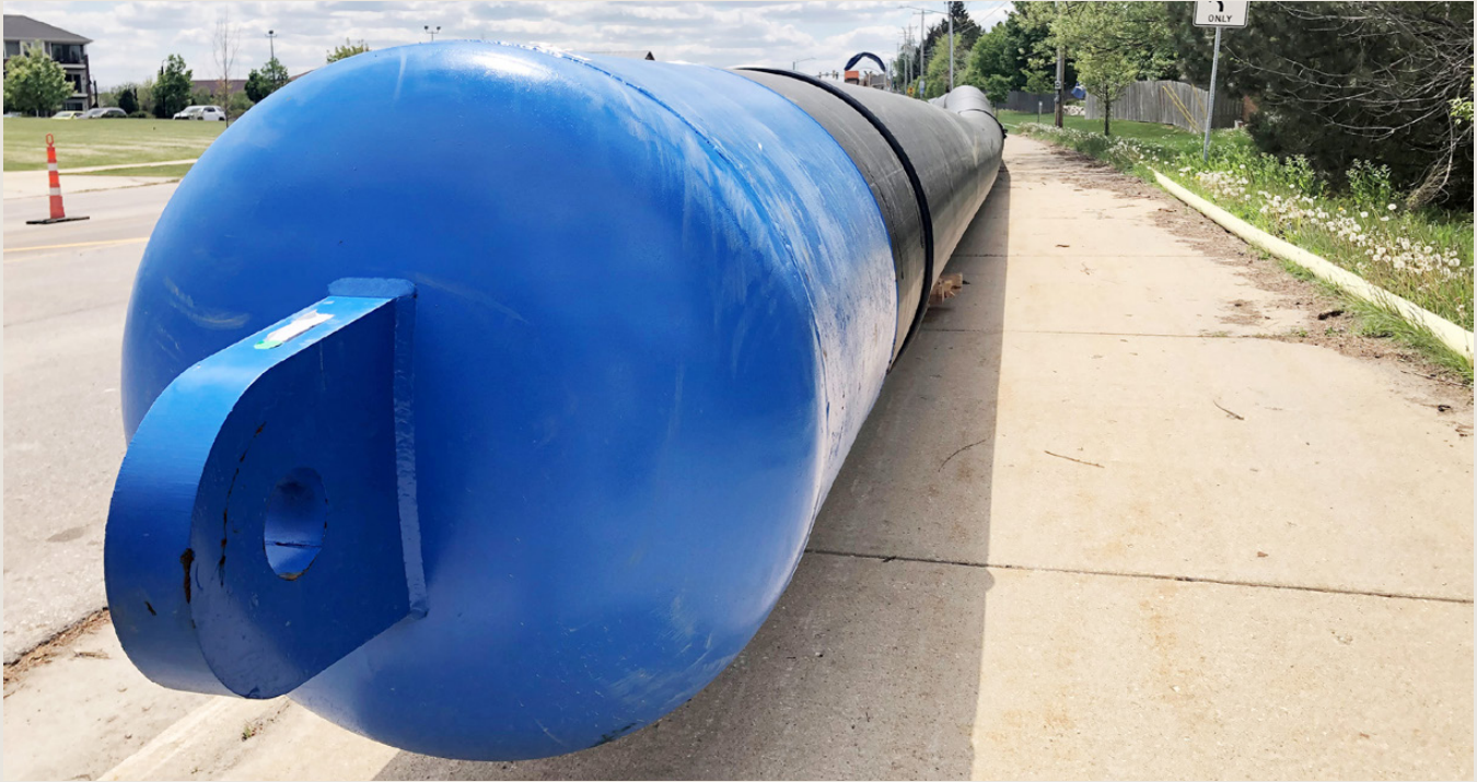
Figure 2. Product pipe ready to go as a larger rig is mobilized to the site
