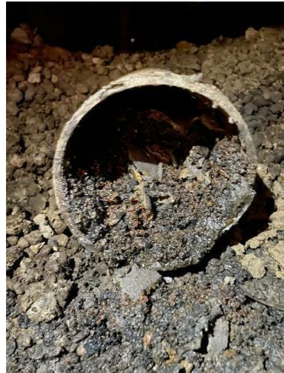
Figure 5. Cleaning Pipes Progressed as Little as 1 Foot Over Several Hours with a Low-Powered Jetter
