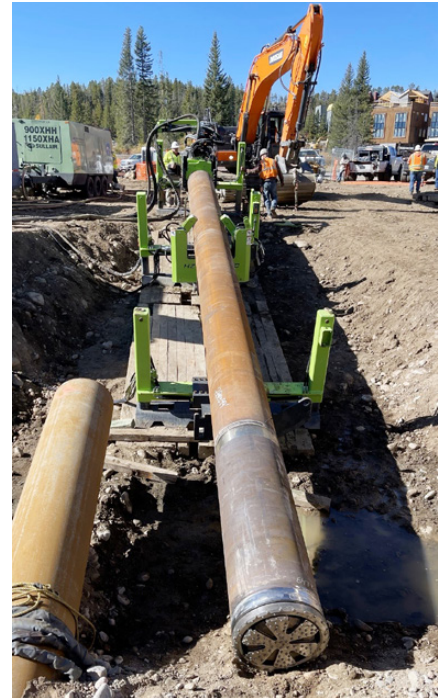
Down the Hole (DTH) Horizontal Hammer Boring was selected as the best method to install the 300 feet of 24-inch conductor casing
