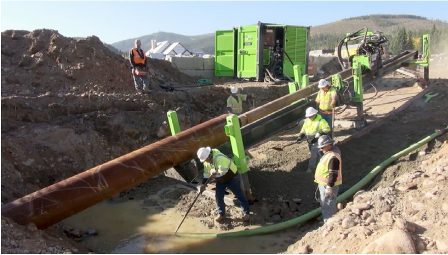
Geonex allowed the contractor to install the conductor casing twice as long as traditional hammer boring methods
