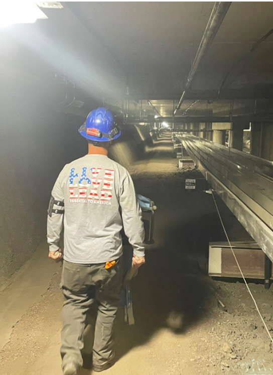
Figure 3. A Maintenance Level below the Tug Tunnels, Enabling Project Crews to Access the Pipe from Narrow Recesses along the Side
