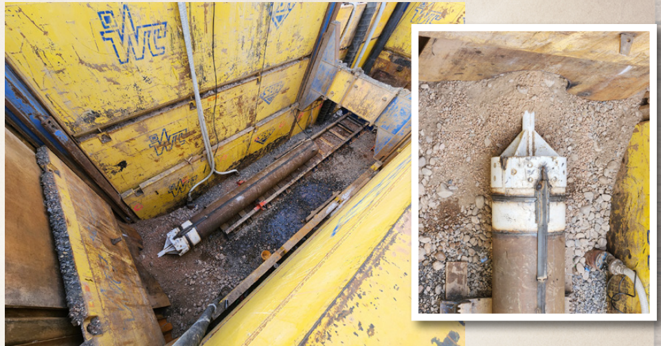
Figure 7. The 4.5-inch to 30-inch step-up adapter just prior to the start of pipe ramming
