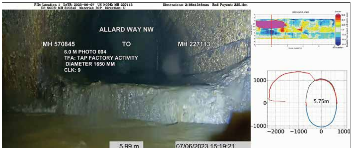
Image shows combined CCTV, LiDAR, and sonar data. All data is tied to the payout. This image shows a large tap in the side of the pipe
