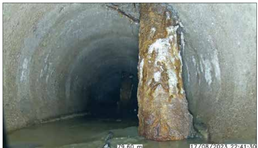
This image shows a pile driven through a Reinforced Concrete Pipe. It shows the perils of not knowing where the underground pipes are. A Pipe Meander Survey may have helped.
