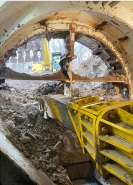
Tunneling Out – the Iowa Trenchless Excavator Shield operator gets a glimpse of their team member operating another excavator
