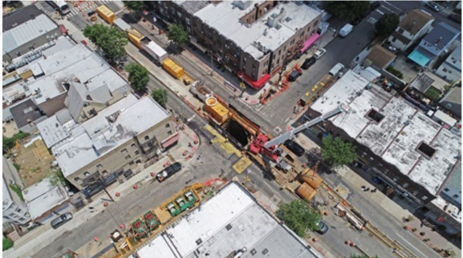
Figure 2. Aerial view of Grand Avenue Jacking shaft and work zone support equipment layout.
