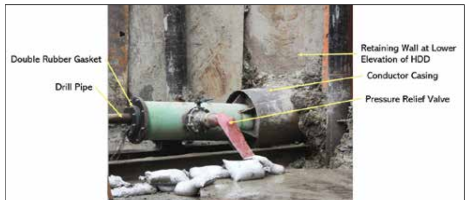
Figure 1. Field-manufactured Packer for maintaining drilling fluid in the borehole during the pilot bore
