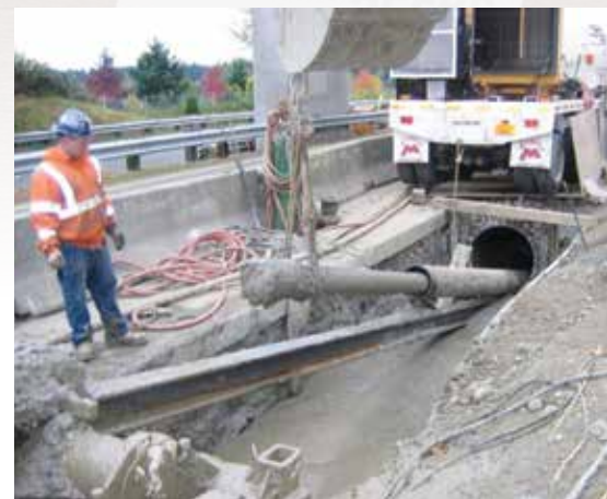
Figure 7. Exit of the pilot bore into the grouted conductor casing used to cut off perched groundwater
