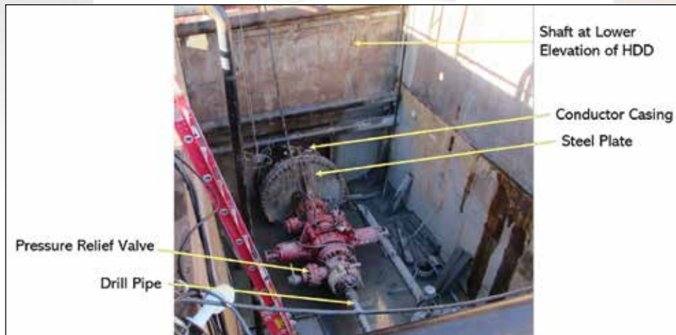
Figure 2. Backflow preventor used to maintain drilling fluid in a gravity HDD with a 40-ft elevation difference between the entry and exit location
