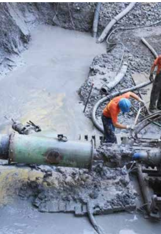
Figure 3. Mud loss at the downstream entry location due to packer unable to maintain adequate pressure in the borehole
