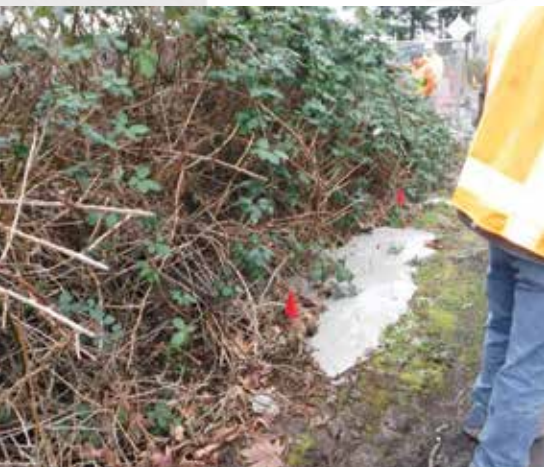
Figure 5. Inadvertent Drilling Fluid Returns at a ditch line when drilling was taking place from the upper end of the bore with over 140-ft of elevation difference
