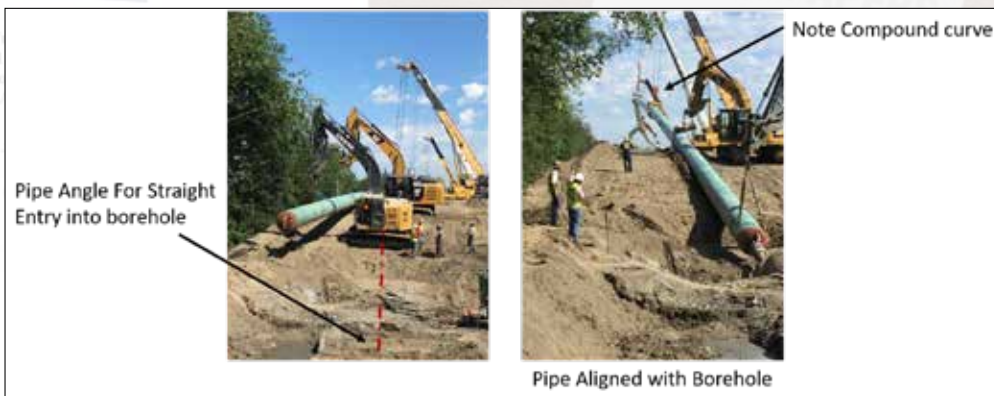
Figure 10. Pulling pipe into alignment for pull-back results in overstressing the pipe at the compound curve
