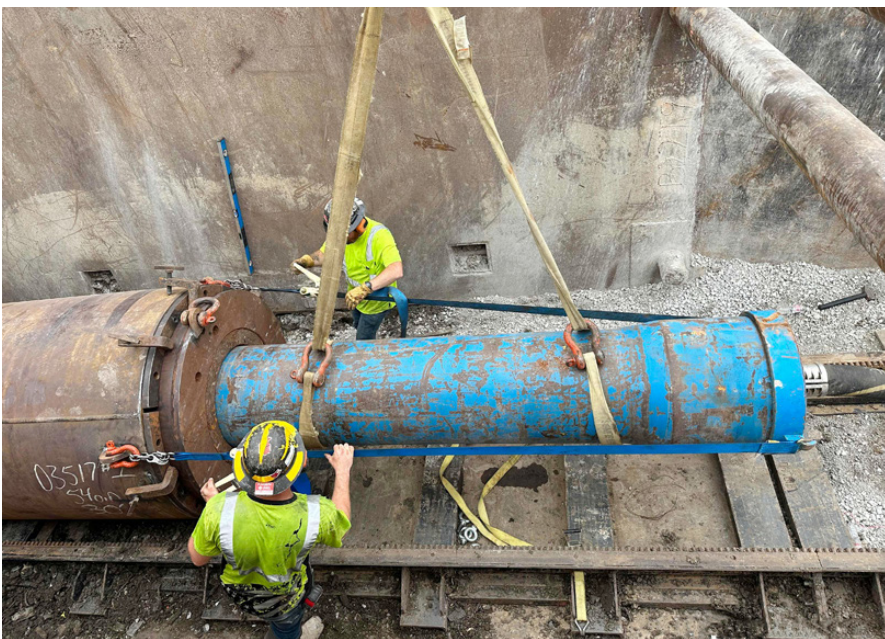
The project in Fort Worth consisted of the installation of two 54-inch conductor barrel pipe rams. The first one was 90 feet, and the second one was 180 feet
