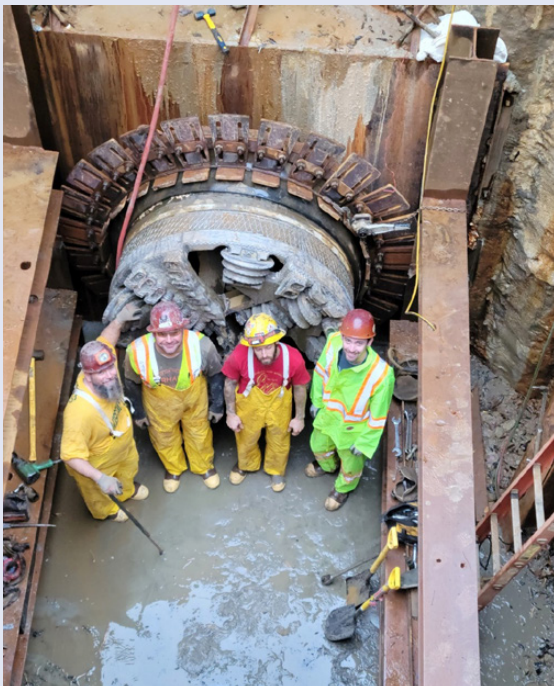
Project entailed the installation of 2516 lf of 48-inch RCP by slurry microtunneling
