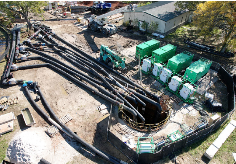
Over 1000KW of temporary generators were used to power the pumping system
