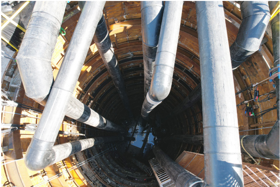
A 65 foot deep shaft was built to house the temporary wet well
