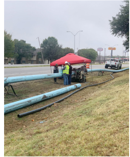
5,100 LF of cast iron (CIP) 12-inch water main was replaced along the 4-line Texoma Parkway
