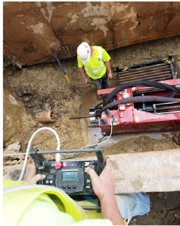
Enhanced safety. Some modern pulling machine designs free the operator from the pit, offering a superior view of the operation and of worksite surroundings during an installation
