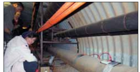
Sepideh Yazdekhashti, a Ph.D. student in the Clemson Department of Civil Engineering, and Josiah Hester, a Ph.D. student in the Clemson School of Computing, work together to collect data by attaching a vibration sensor to a 10-in. cast iron water pipe in a Clemson campus tunnel.
