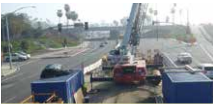
Figure 2 – View down the tunnel alignment from the launch shaft on Pacific Coast Highway.
