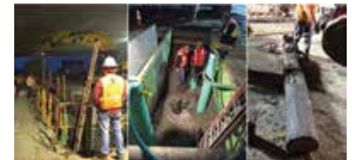
Figure 4 – Pile obliteration trench (left); exposed battered timber pile tips (middle); timber pile (right).
