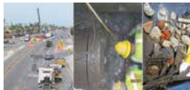
Figure 3 – Rescue shaft (left) to remove reinforced concrete obstruction (middle) and debris (right) from tunnel alignment.
