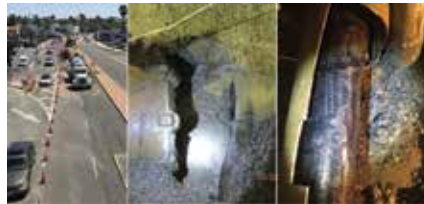
Figure 5 – Rescue shaft in the middle of Pacific Coast Highway (left) to access the MTBM that indented the steel casing (middle) housing the high-pressure gas main (right).
