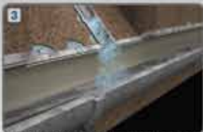
Continues to leak in annular space
