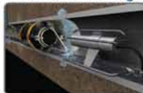
Leaking joint in mainline sewer
