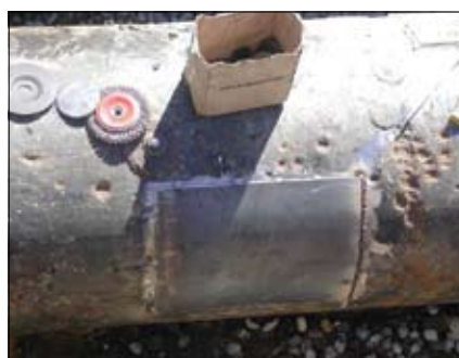
Figure 2. Condition of the pipe found. Note the patch to fix the leak.
